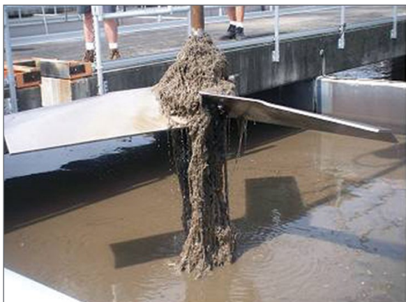
HE-3 impeller ragging after eight weeks in operation at a Florida wastewater treatment facility
